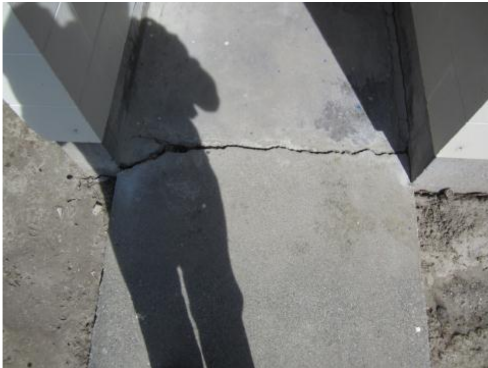
Photograph 4 Cracking in concrete floor slab at the eastern corner of the building
