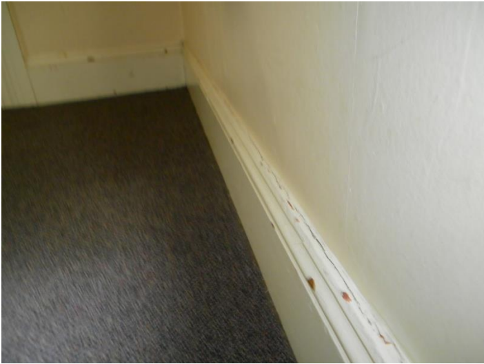
Lining damage at floor level
