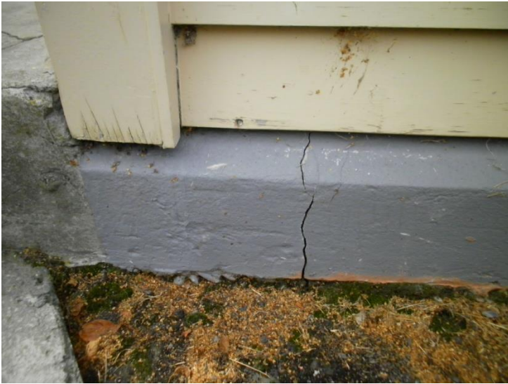
Crack in concrete perimeter foundation
