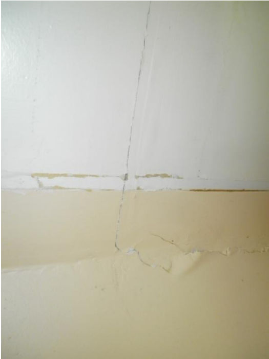
Lining damage at ceiling wall intersection
