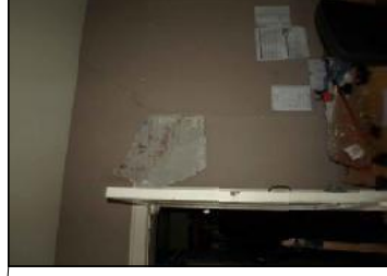
damage to wall in office
