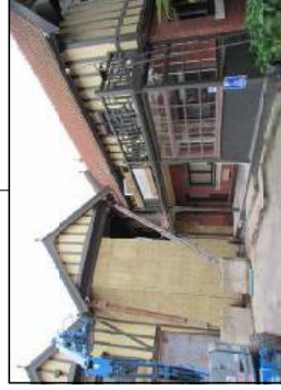
damage to wall around stair lobby
