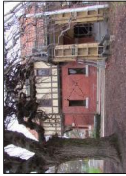
damage to walls to drawing room
