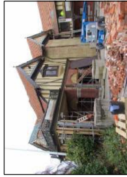
damage to columns to patio area
