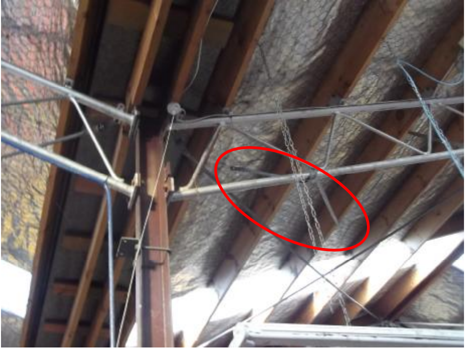
Photo 5: Damaged fly brace
