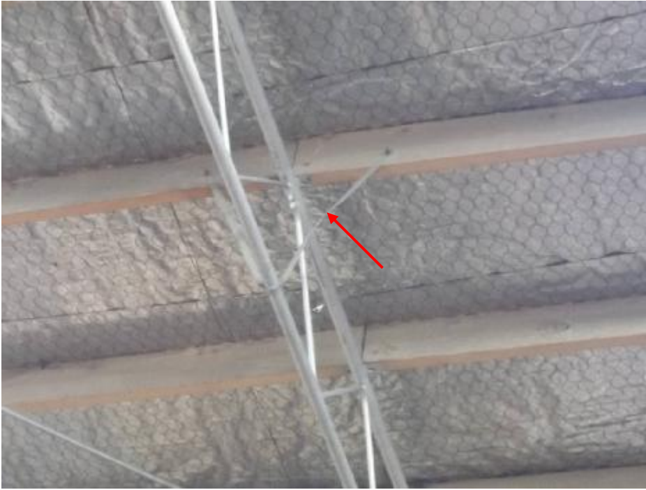
Photo 4: Damaged fly brace
