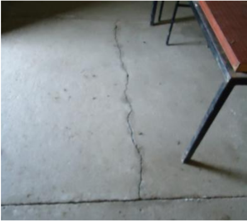
Photograph 5 Cracking to slab.
