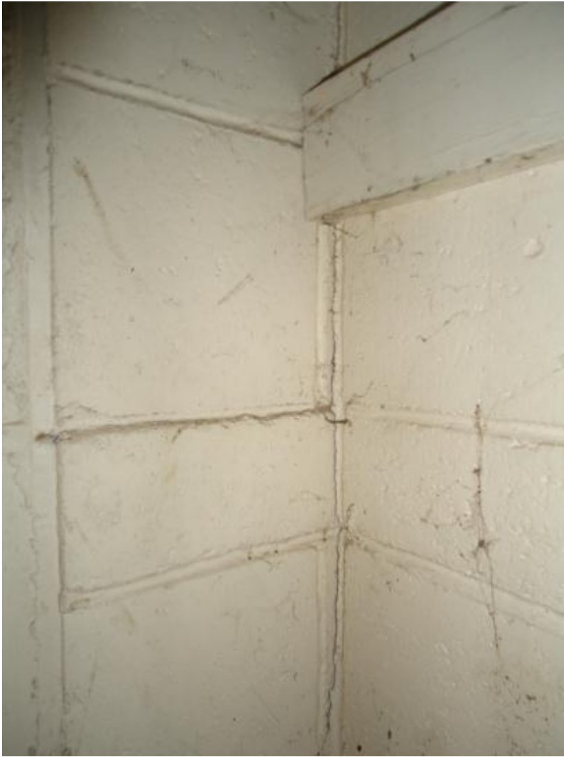
Photograph 6 Cracking to block wall at connection.
