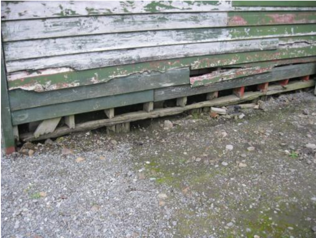
Photograph 3 Rotten timber piles and timber bearer, and broken weatherboards.
