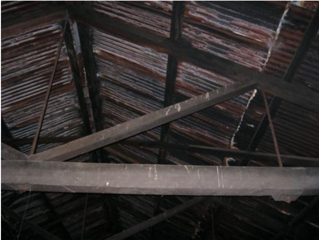
Photograph 5 Timber truss roof structure with rusted corrugated iron cladding above.
