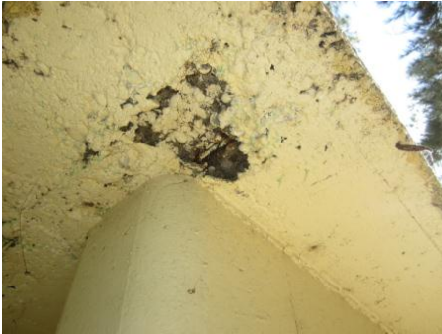
Photograph 5 Example of minor spalling in concrete roof slab
