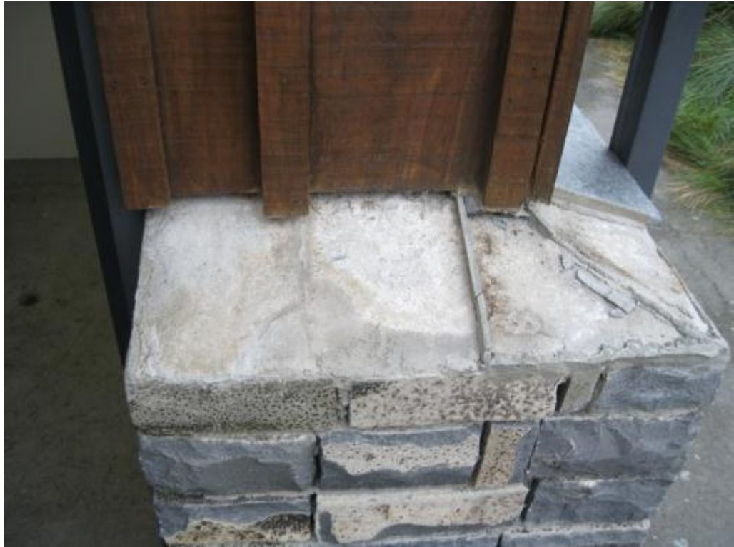
Photograph 5 Missing tiling on stone veneer
