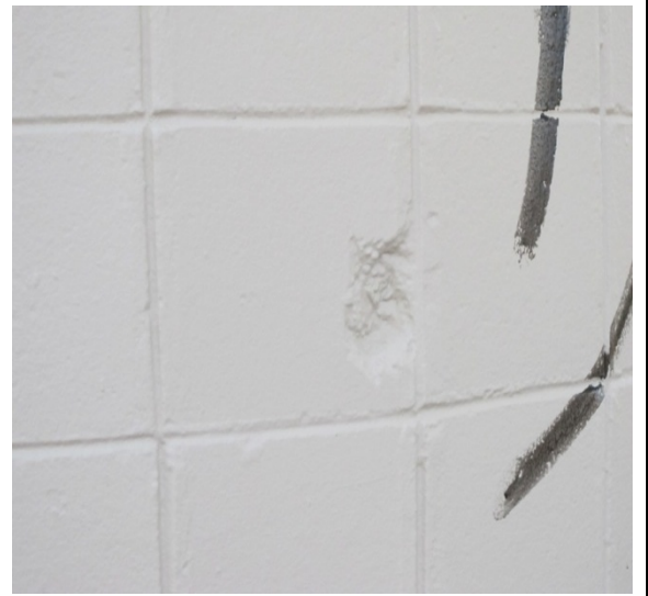
Photo 6: Impact damage on west wall.
