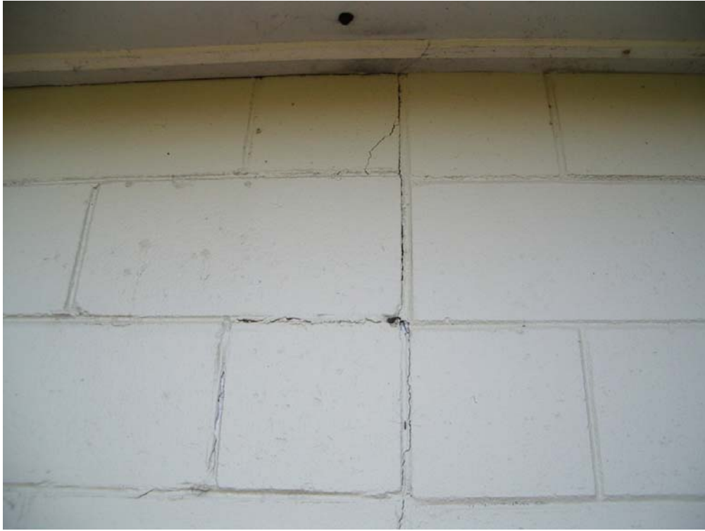
■ Figure 9 Minor cracking observed
