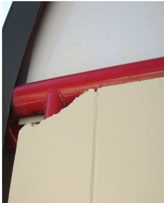
Photo 11: Impact damage to top of masonry wall above west toilet entrance.
