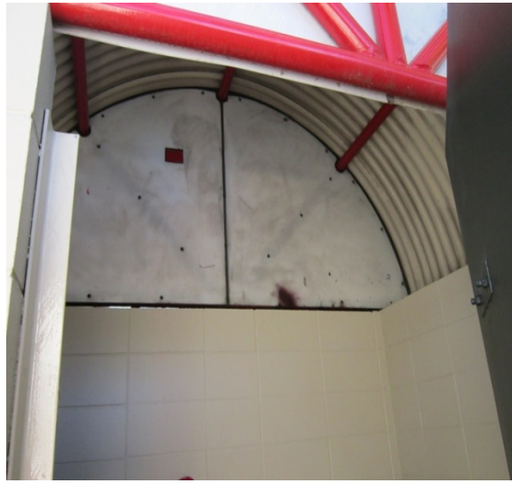
Photo 9: Internal masonry wall between the east and west toilets. Steel roof framing also shown.
