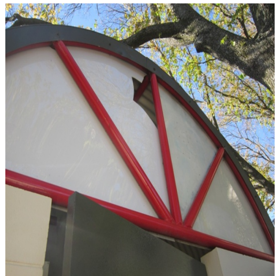
Photo 14: Impact damage on roof cladding above west toilet entrance.
