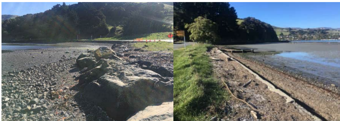
Figure 4.37: Example of protection structures with evidence of scour and overtopping (Duvauchelle Bay).
