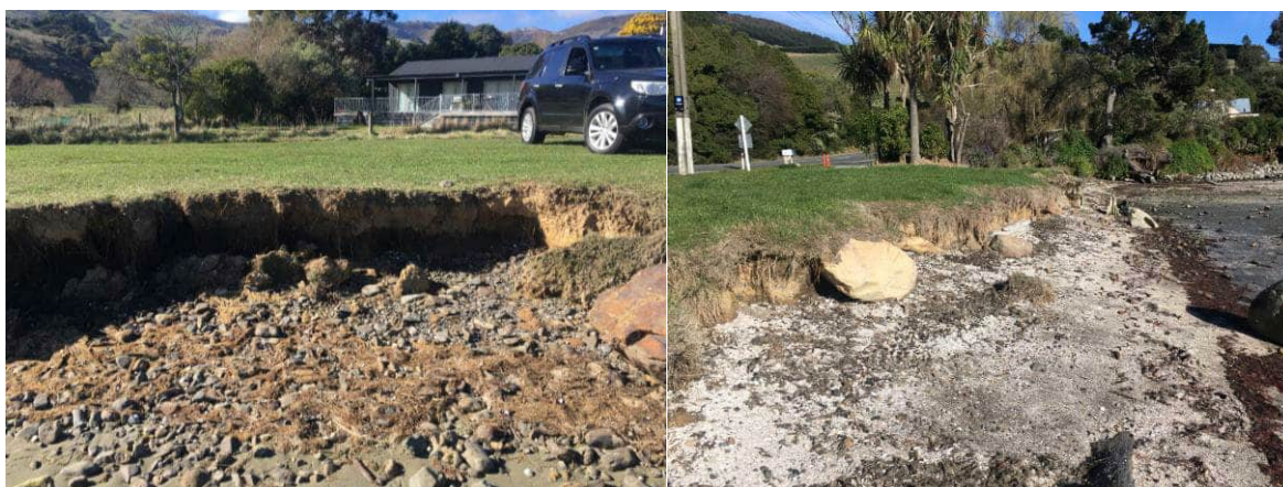
Figure 4.38: Example of unprotected eroding harbour shorelines. (Left) Takamatua Bay, (right) Charteris Bay.
