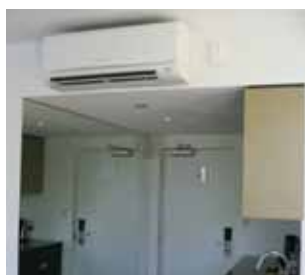
Heat pump in guest room © Copyright
