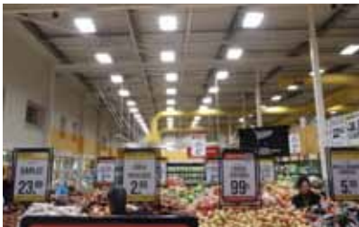
New shop floor T-5 tubular fluorescent bulbs © Copyright
