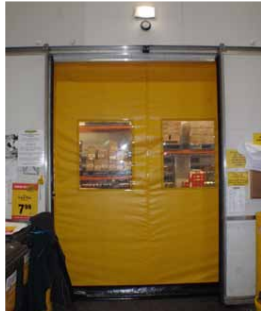
Automatic chiller door © Copyright
