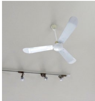
High level fan moving air to occupied level © Copyright
