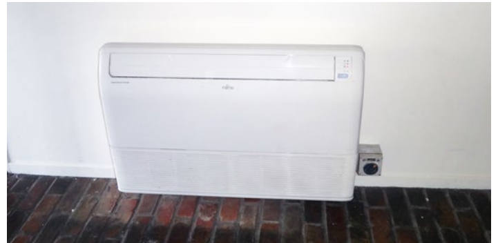
One of several heat pumps installed © Copyright
