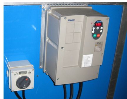
Variable speed drive on one of the AHUs © Copyright
