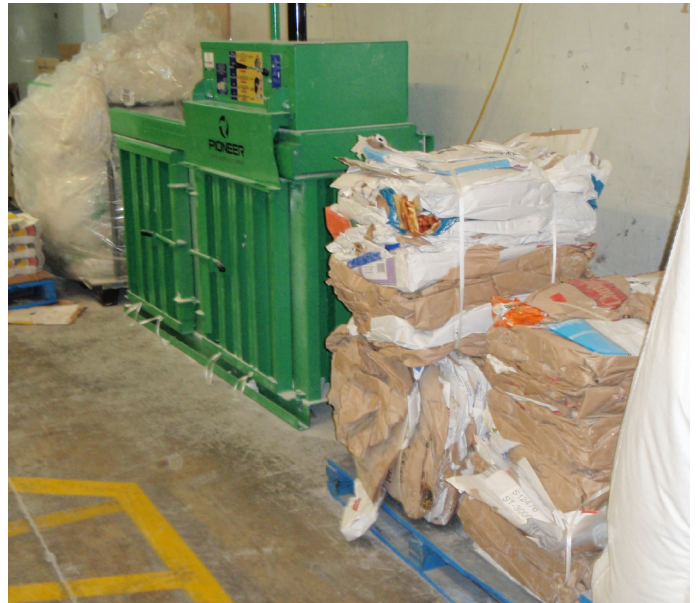
Cardboard and plastic baling machine installed to pack the cardboard and plastic ready for recycling © Copyright
