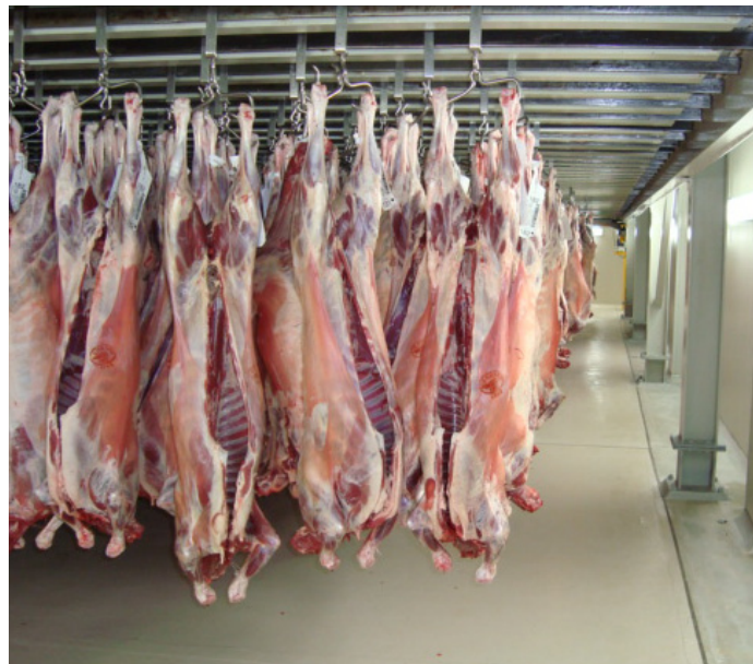
Chiller area © Copyright
