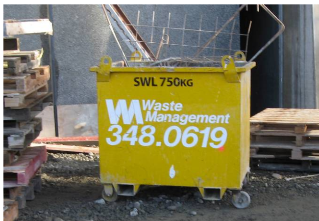
Bucket skips used to transport waste to the central sorting area © Copyright
