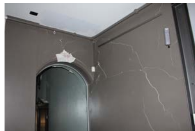
Typical plaster damage to ground floor masonry walls.
