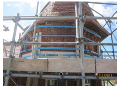
The turret to the south-east corner showing the displacement of the roof towards the east.
