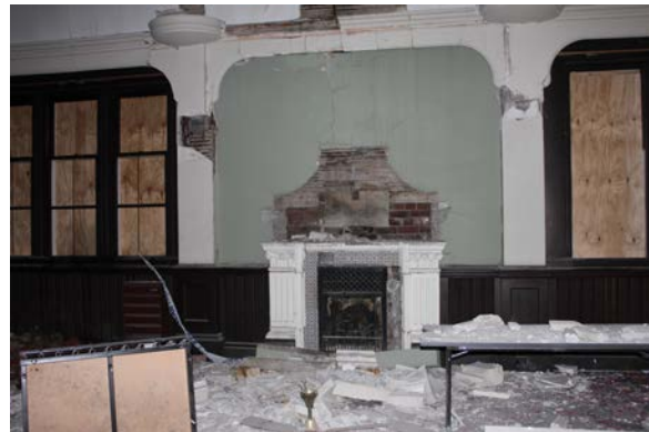
The partially collapsed fire surround and over mantle of the west fireplace in the Chamber following the February 2011 earthquake.
