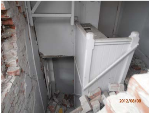
North-west stairwell damage and collapsed walls.
