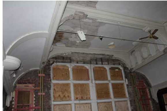
The Council Chamber, south window and wall. The inner wythe of brick collapsed exposing the rear of the figurines either side of the window and the plaster render collapsed off the wall in its entirety.
