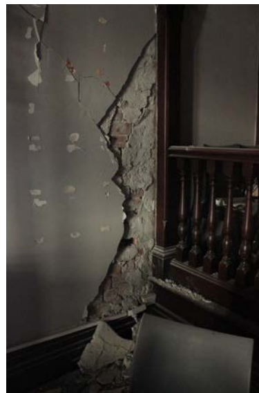
The damaged wall adjacent to the Library arcade balustrade.
