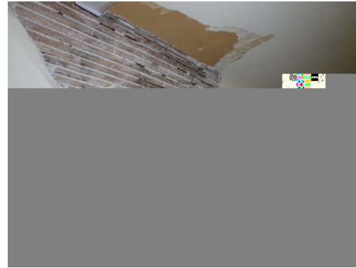
Typical lath and plaster ceiling damage to the second floor attic space ceilings.
