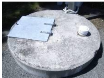
Wastewater Tank/Pump Chamber
