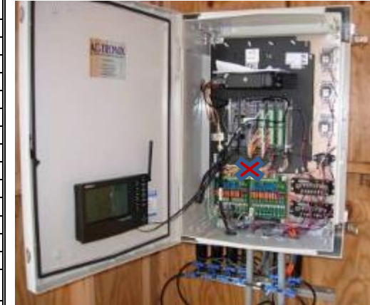
Irrinet system in wall cabinet.
