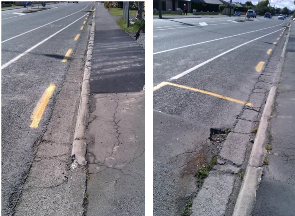
Figure 10-23: Kerb and channel degradation, south side of Sawyers Arms
