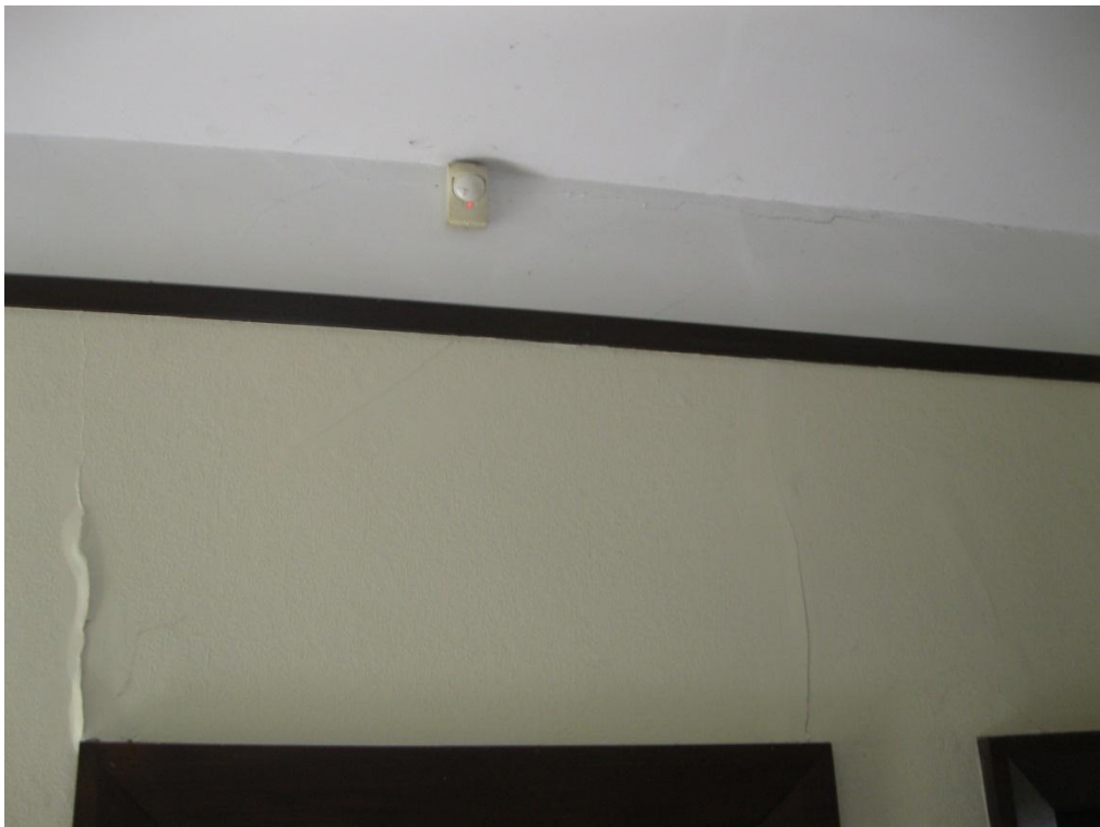
Photograph 6 Vertical cracking in what is likely to be plasterboard wall lining.
