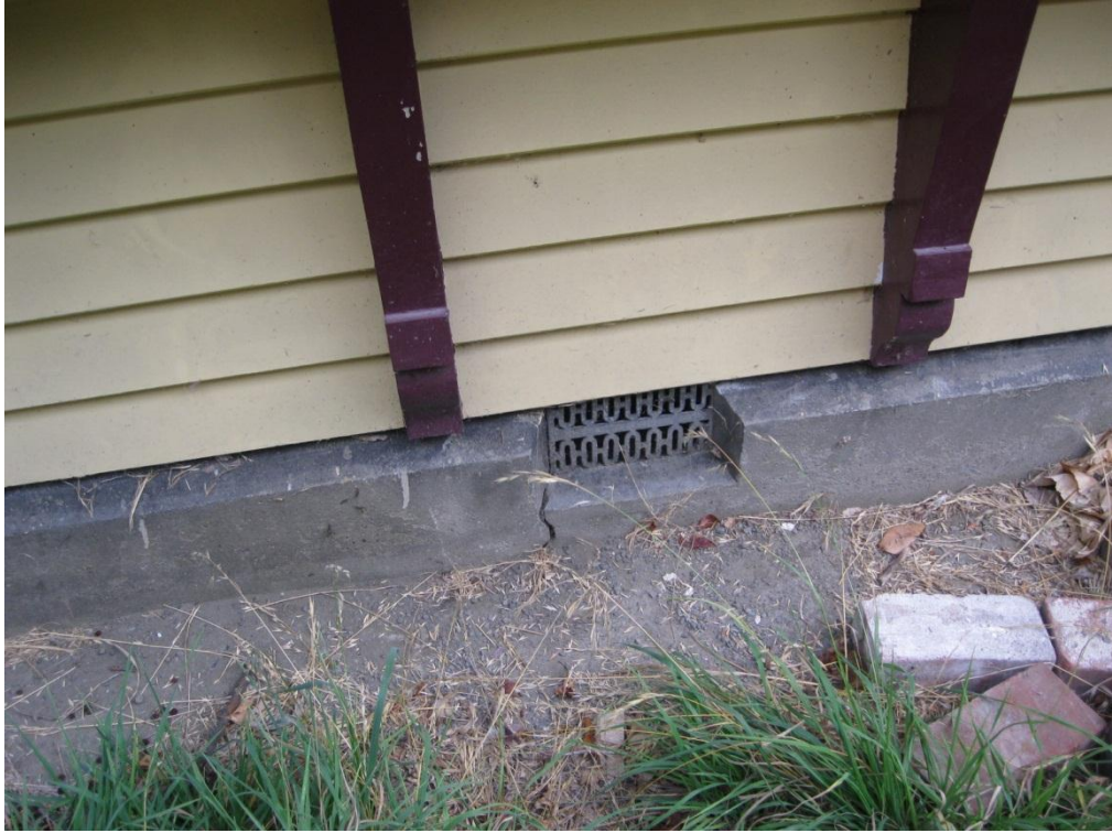
Photograph 11 Cracking to concrete perimeter strip foundation.
