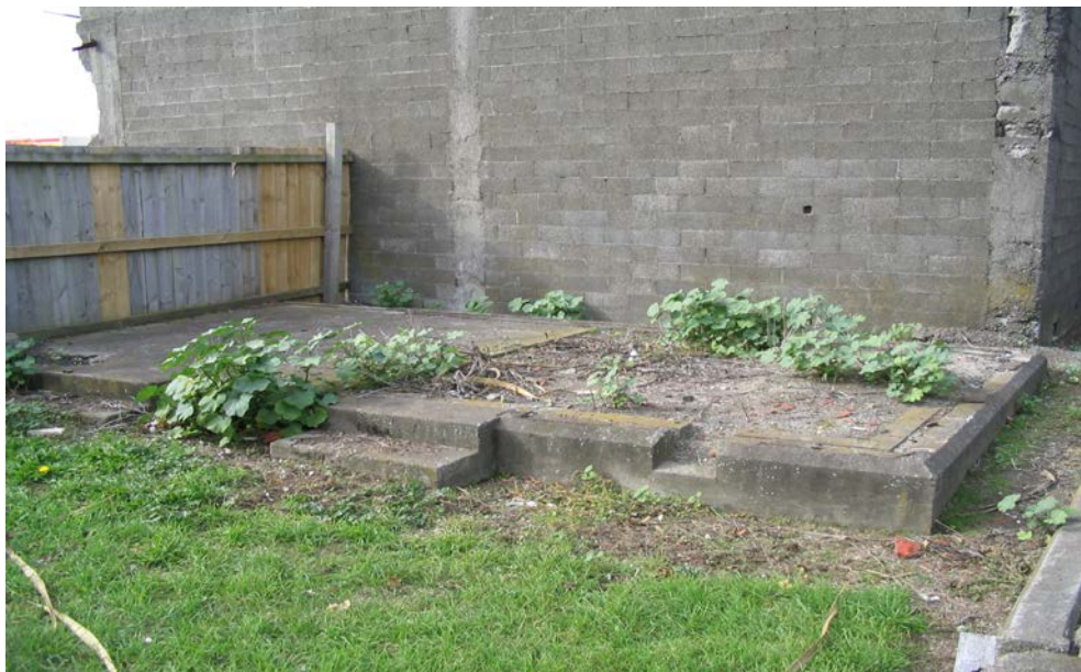
Likely foundations of the Sextons office and tool shed as noted in the Building Permit of 1923 and 1947 Reserves Committee report.
